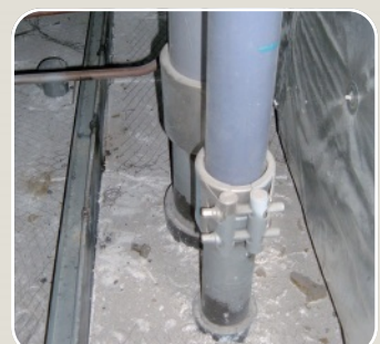
▲ PVC + Steel Pipe Connection
