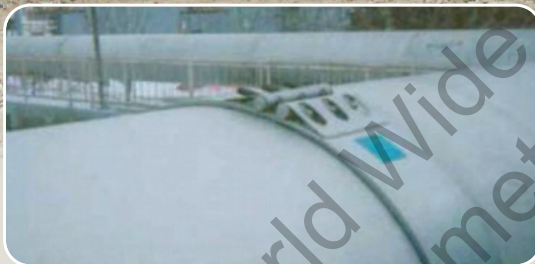
▲ 48" (1,200A) YNMF-RL Canadian power plant cooling line
