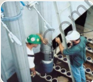
▲ Canada: water purification facility
