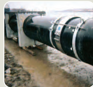
▲ U.S.: nuclear power plant
