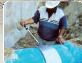
▲ UK: buried water supply pipes
