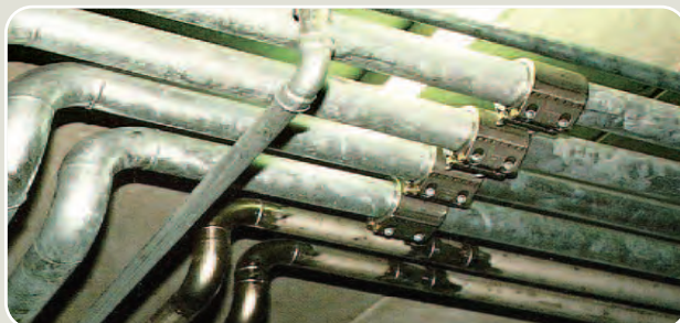
▲ Water supply pipes with an apartment house BIT
