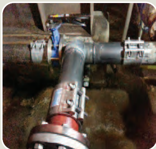
▲ Netherland desalination treatment facilities
