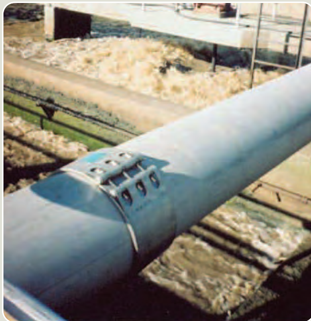
▲ Spain: water purification facilities
