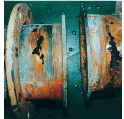
DAMAGES OF A COPPER NICKEL PIPE AFTER SIX
